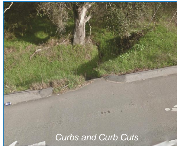
Catch Basin and Storm Drain System
