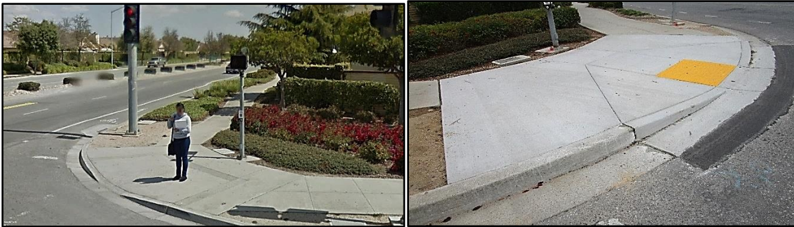
Before and after photo of ADA Pedestrian Ramp at N Sanborn Rd and Freedom Pkwy
