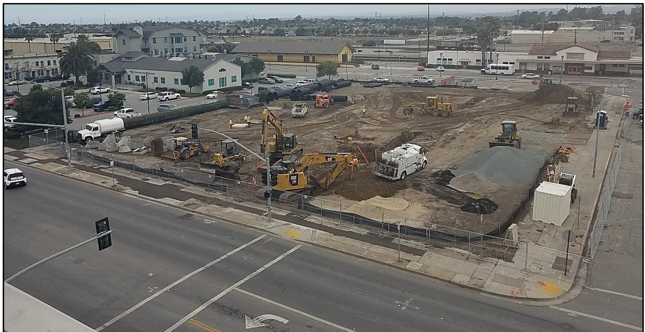
Demolition of existing structures north of Lincoln Avenue and west of Station Place
