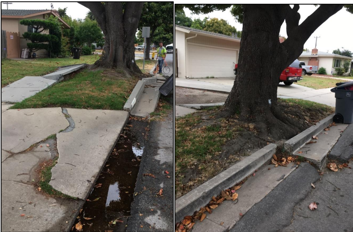
Before photos of Central Ave JOC Sidewalk Repair
