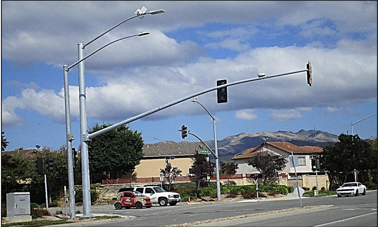
(After) New Traffic Signal with Protected Left-Turns at N Sanborn Rd and Freedom Pkwy
