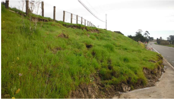
Slipout encroaching onto road
